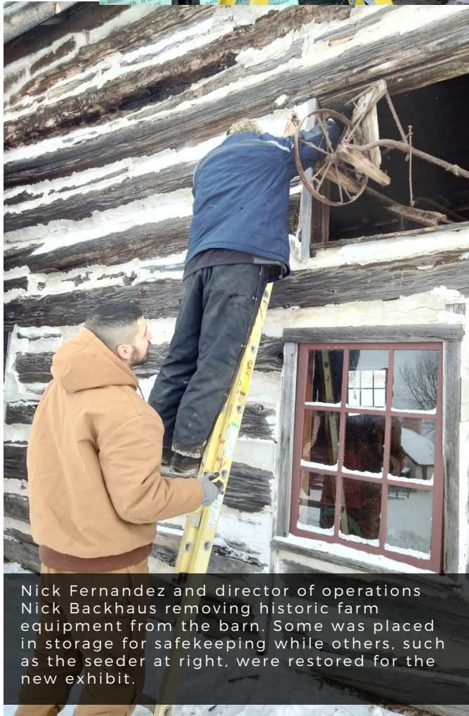
Preservation carpenter and maintenance tech. David Haack, assisted by Nick Fernandez, installing signage and the restored farm equipment.
